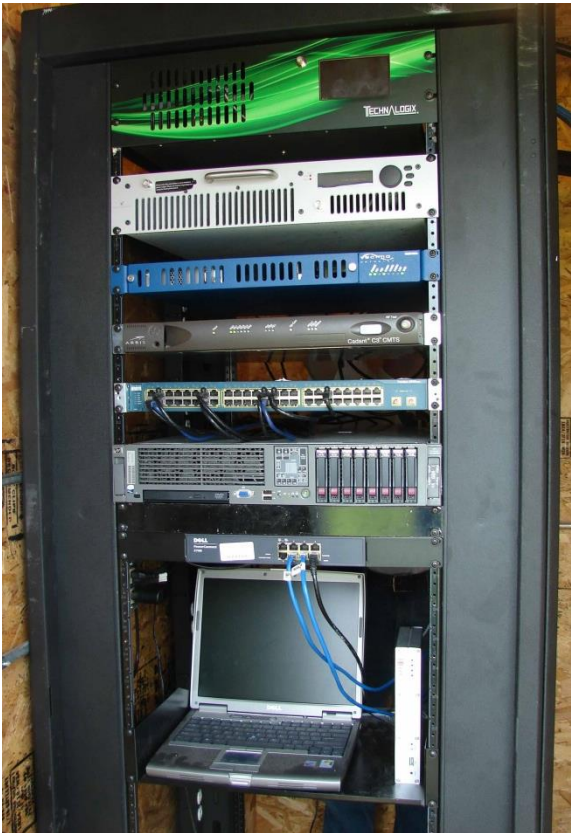
Rack of Base Station Equipment
